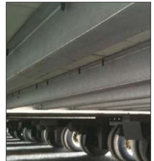
Truck trailer beams are exposed to a variety of harsh conditions.
