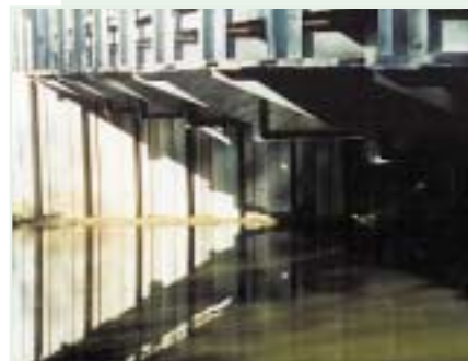
View of north end wall abutment and partial view of bridge underside
