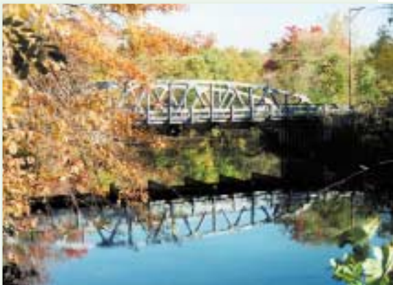
This fully galvanized truss bridge is performing well after five years of service in a moderately industrial corrosive environment. See story on page 2.
