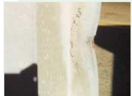
Collision damage to vertical truss chord.
