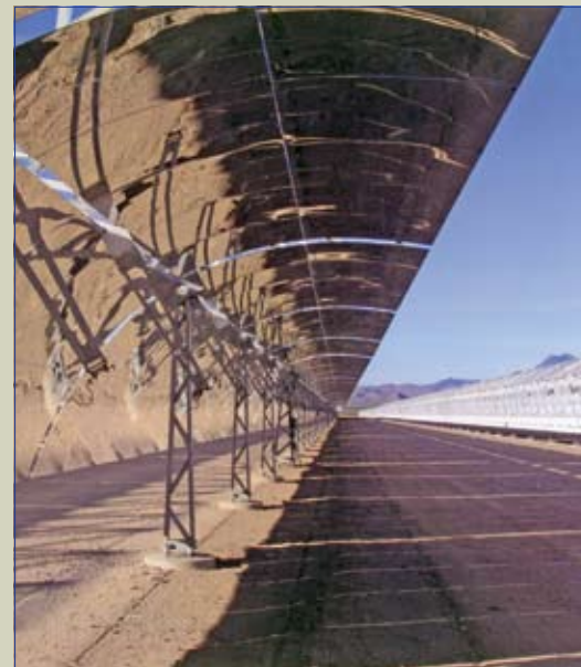
Sixty-four megawatts of power will be generated by the 180,000 mirror panels in the farm.
