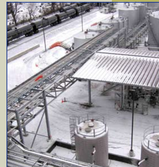
The exposed galvanized steel used in this plant will be protected from harsh snow and rain exposure.
