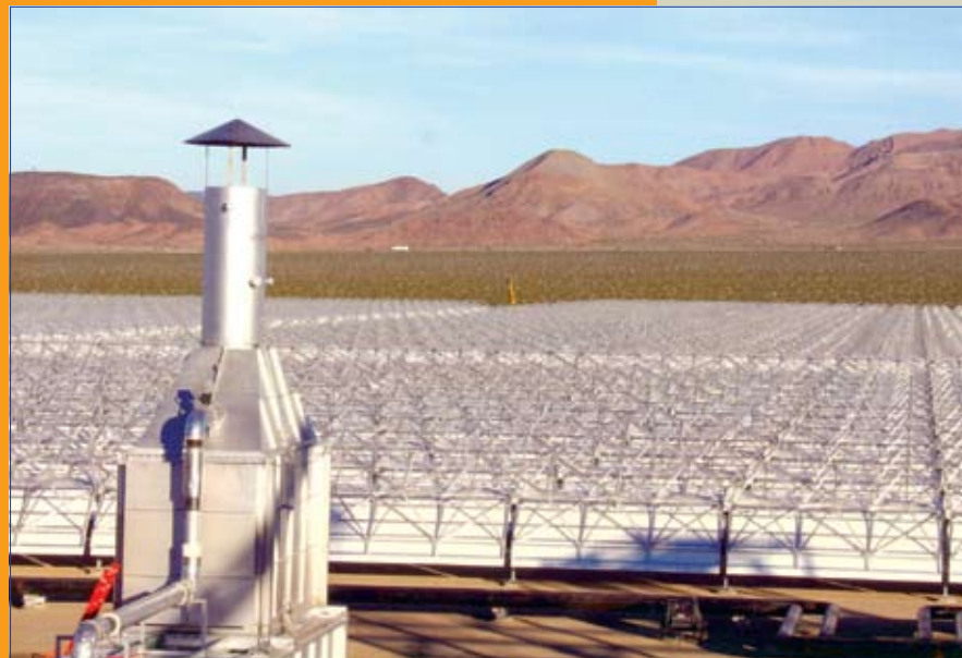
This solar energy farm is the largest capacity facility of its kind built in the past 15 years, spanning more than 400 acres with computer-controlled reflective mirrors.
