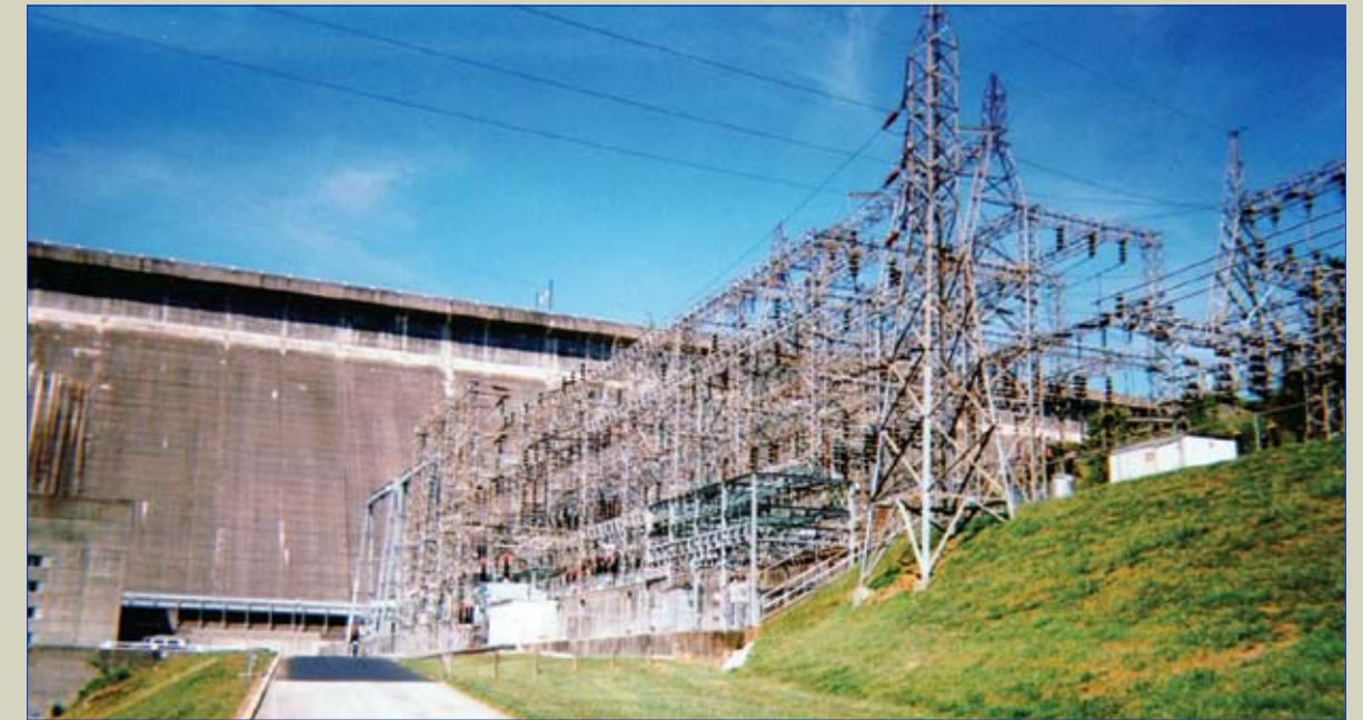
In keeping with the environmentally-friendly purpose of this hydroelectric substation, the Norris Dam Steel Substation was hot-dip galvanized with natural, sustainable zinc for corrosion protection.
