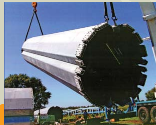
Separating the wind tower into several pieces made it considerably more economical to transport.
