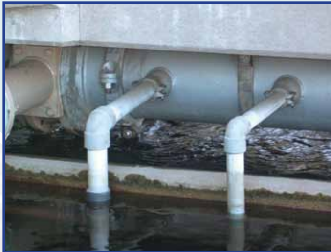
This water treatment facility was galvanized to protect steel from the many corrosive properties of ground water.
