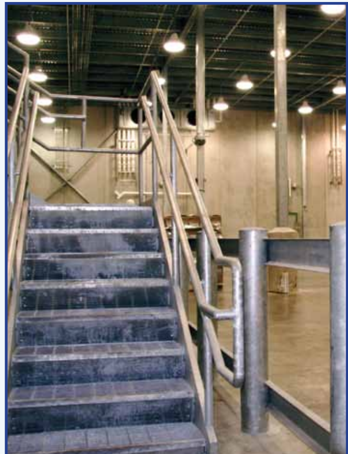
The Quick Chill Cooler expansion was hot-dip galvanized to help meet USDA food processing requirements and to withstand the extreme cold environment.
