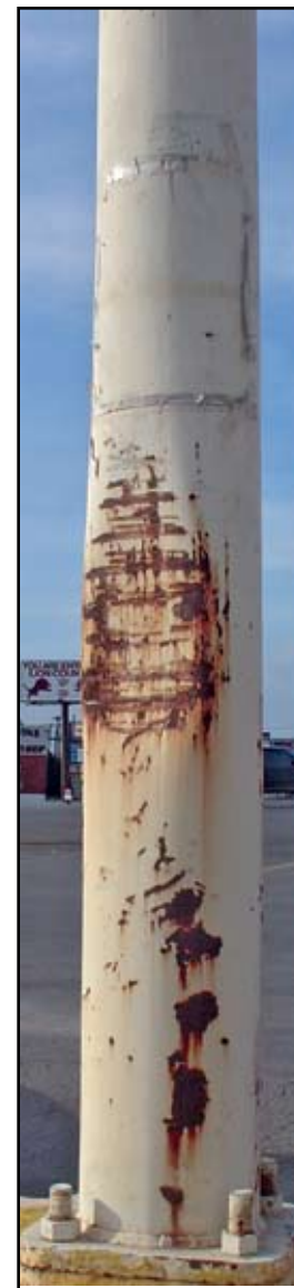
Corroding painted pole
