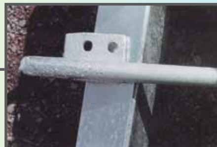
FIGURE 35: WELDING SPATTER (REJECTABLE)
