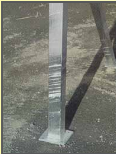
FIGURE 23: OXIDE LINES (ACCEPTABLE)
