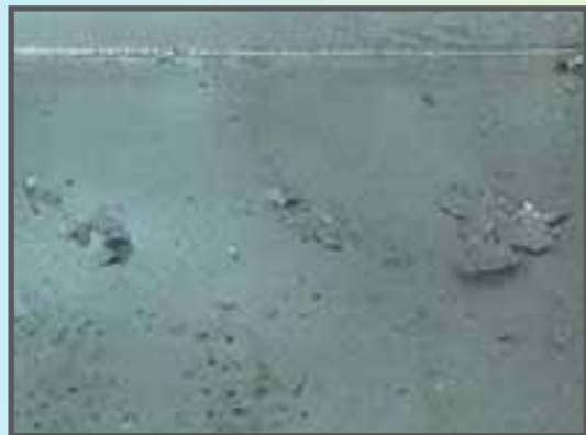
FIGURE 38: ZINC SPLATTER (ACCEPTABLE)
