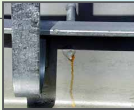
FIGURE 33: WEEPING WELD (ACCEPTABLE)
