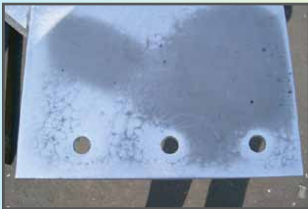
FIGURE 10: GRAY COATING DUE TO TEMPERATURE DIFFERENCES (ACCEPTABLE)
