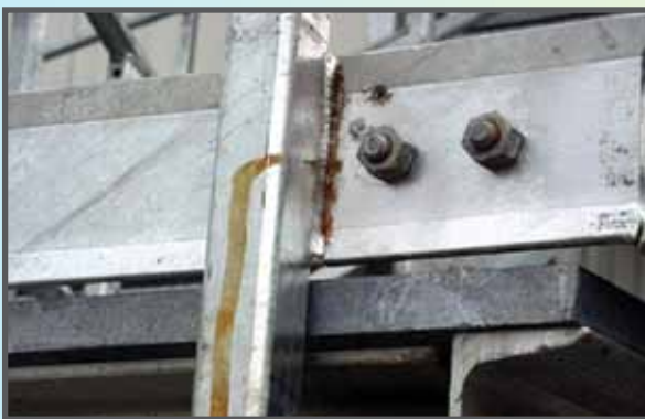
FIGURE 28: RUST BLEEDING (ACCEPTABLE)
