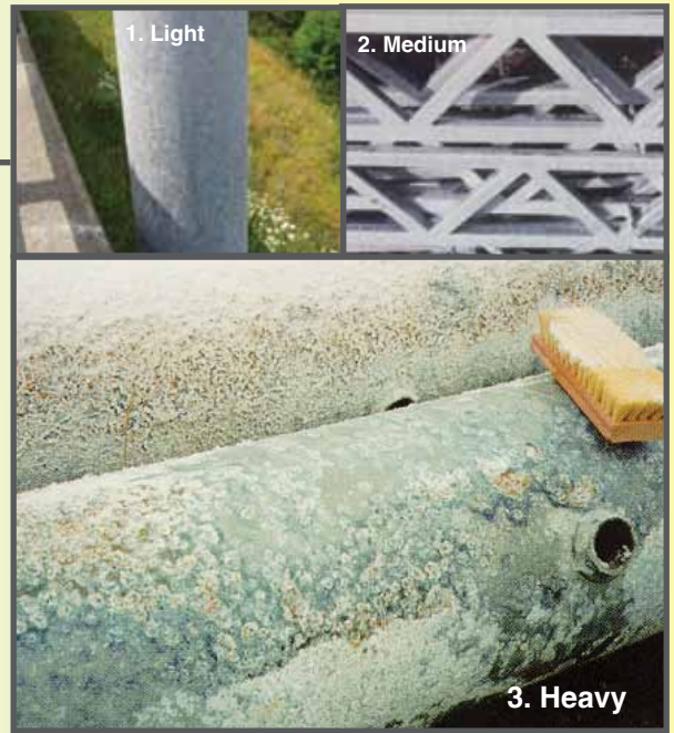
FIGURE 36: WET STORAGE STAIN (LIGHT (1) OR MEDIUM (2) IS ACCEPTABLE, HEAVY (3) IS REJECTABLE)
