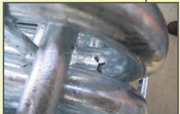
FIGURE 12: BARE SPOTS (REJECTABLE)
