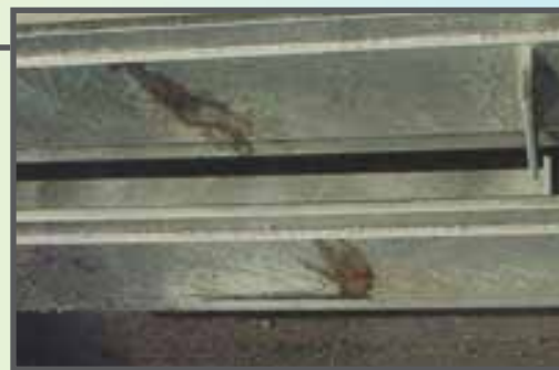
FIGURE 34: WELDING BLOWOUT (REJECTABLE)
