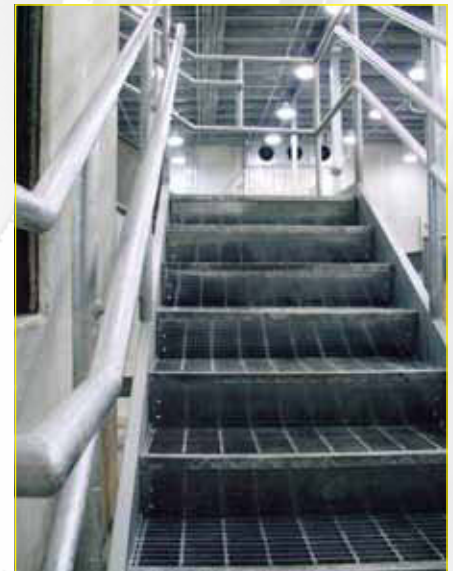
This staircase belongs to the 160,000 square foot Quick-Chill Cooler, a facility that was hot-dip galvanized to protect it from the corrosiveness of chicken and beef processing.
