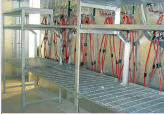
These hot-dip galvanized storage racks in Buffalo Wild Wings are protected from drips and condensation.
