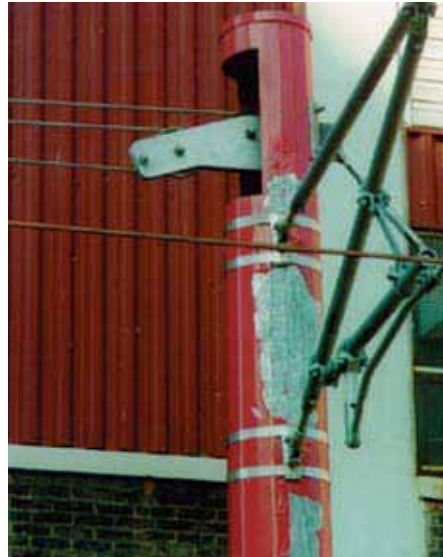
Peeling paint from untreated galvanized pole
