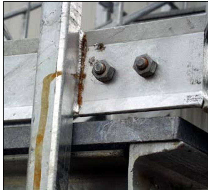
Rust bleeding results from the interaction of moisture, cleaning chemicals, and uncoated steel surfaces where a full seal weld was not achieved during the design/fabrication phase.
