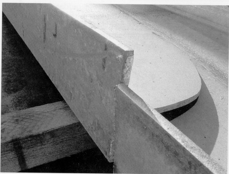
Figure 2. I-Beam with web and flange crack.
