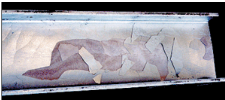
Flaking of a galvanized coating
