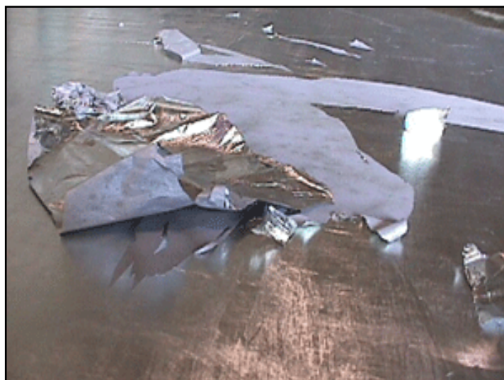
Peeling of a galvanized coating
