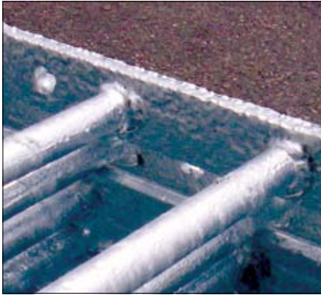
Figure 1: Rough surface due to excessive silicon content
