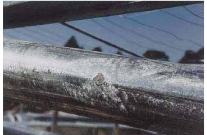
Figure 2: Touch marks on a hot-dip galvanized product.
