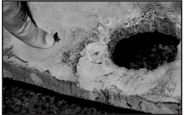
Figure 1: Kettle Perforation Failure
