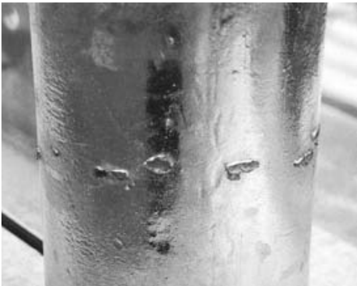
Figure 1: An example of chain marks caused during HDG.
